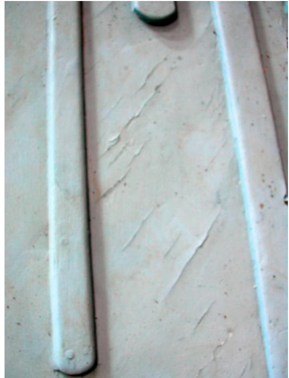
A124 Helene, deck degradation, 2008
