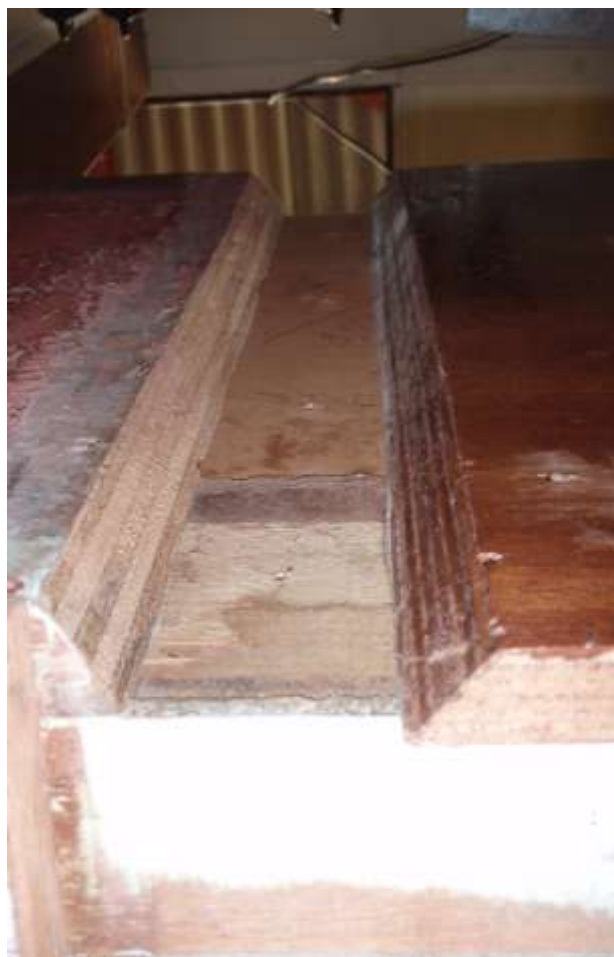
Looking up the joint ready for the fillet to be fitted. Note the poor quality of ply used in the original construction compared to the replacement.
