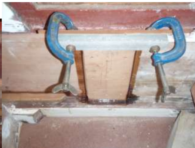
The doubler screwed and resined in position whilst the alignment of the joint is maintained with clamps. Note: - The next section of the 1"x1" fillet will be recessed to bridge the doubler.
