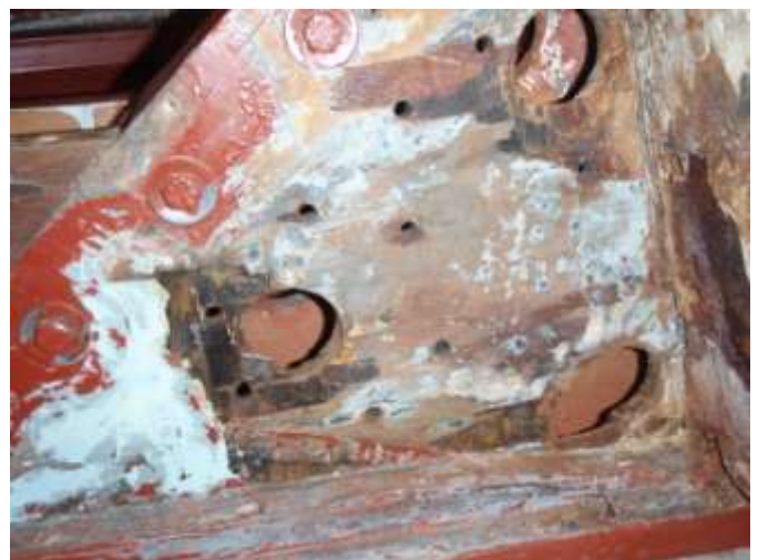
The damaged keel box side. Note the damage to the diagonal bulkhead
