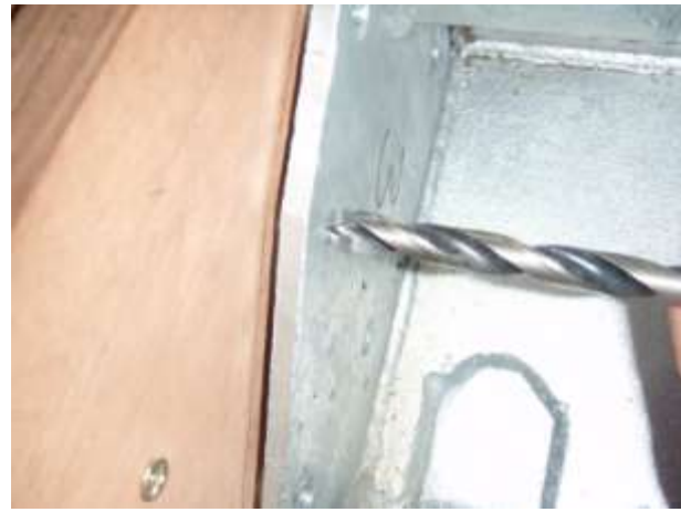
Marking the bolt holes. Note the gap where a cork gasket fits.
