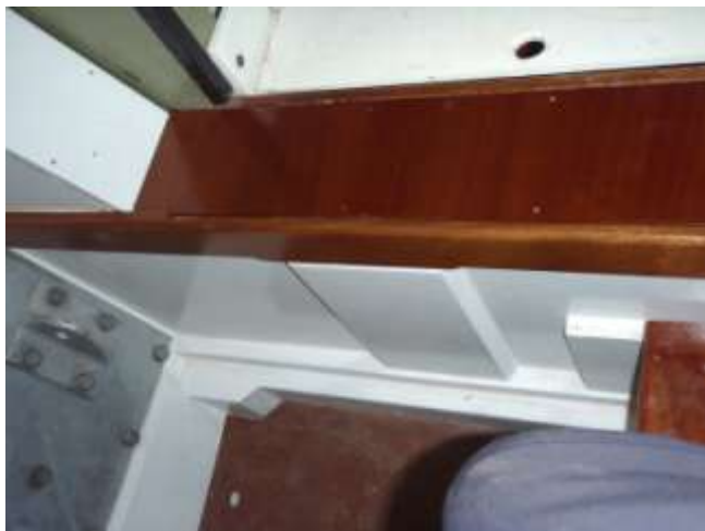
Job done. Note the block below the backing plate that locates the doubler.
