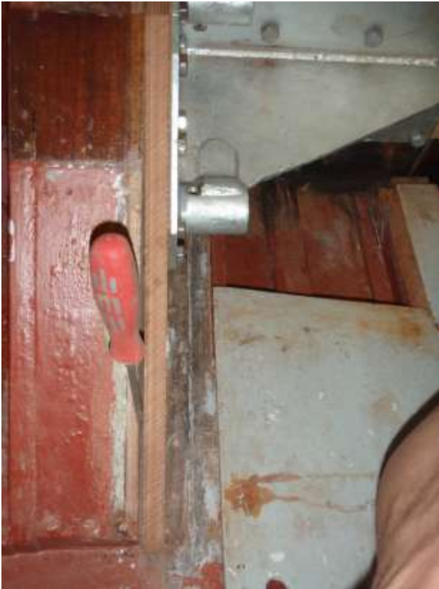
The new keel box side in position. Note the gap that needs a fillet and filler between it and the forward keel block.
