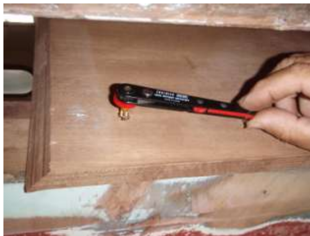
A mini-wrench being used to screw the new keel box side in place
