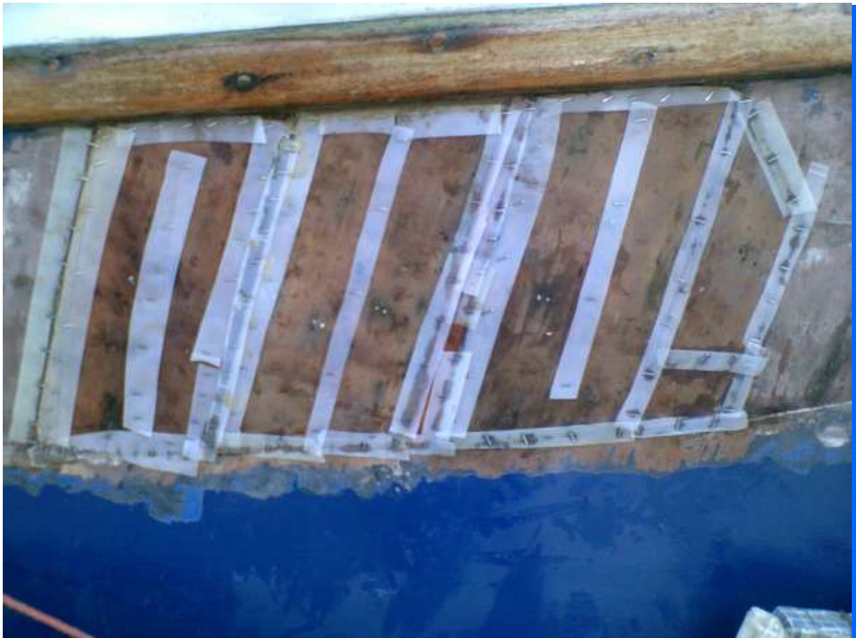
The repair stapled up
