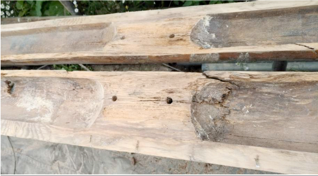
Figure 12 Spreaders area – internal view of damage.
