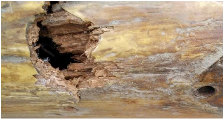
Figure 11 Spreaders area – external view of damage.
