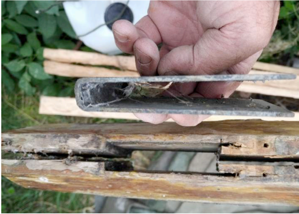
Figure 7. Main Halyard sheave fitting removed.
