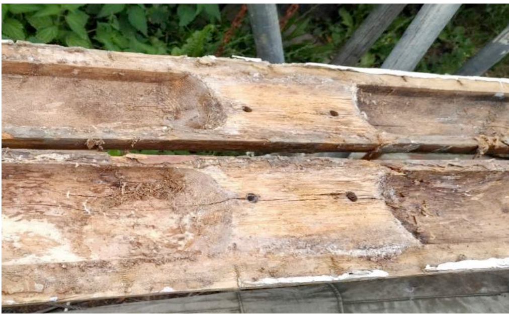
Figure 10 Diamond brace area – internal view of damage.
