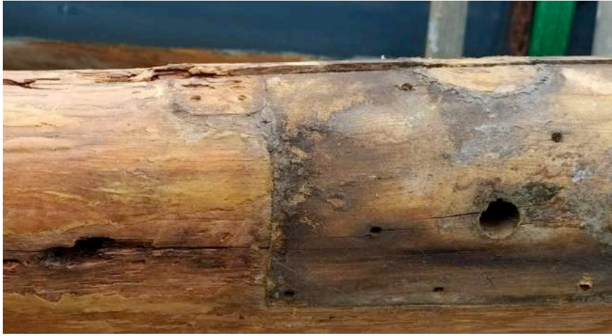
Figure 9 Diamond brace area – external view of damage
