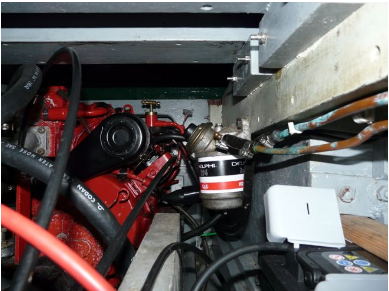
New fuel filter with lift pump attached
