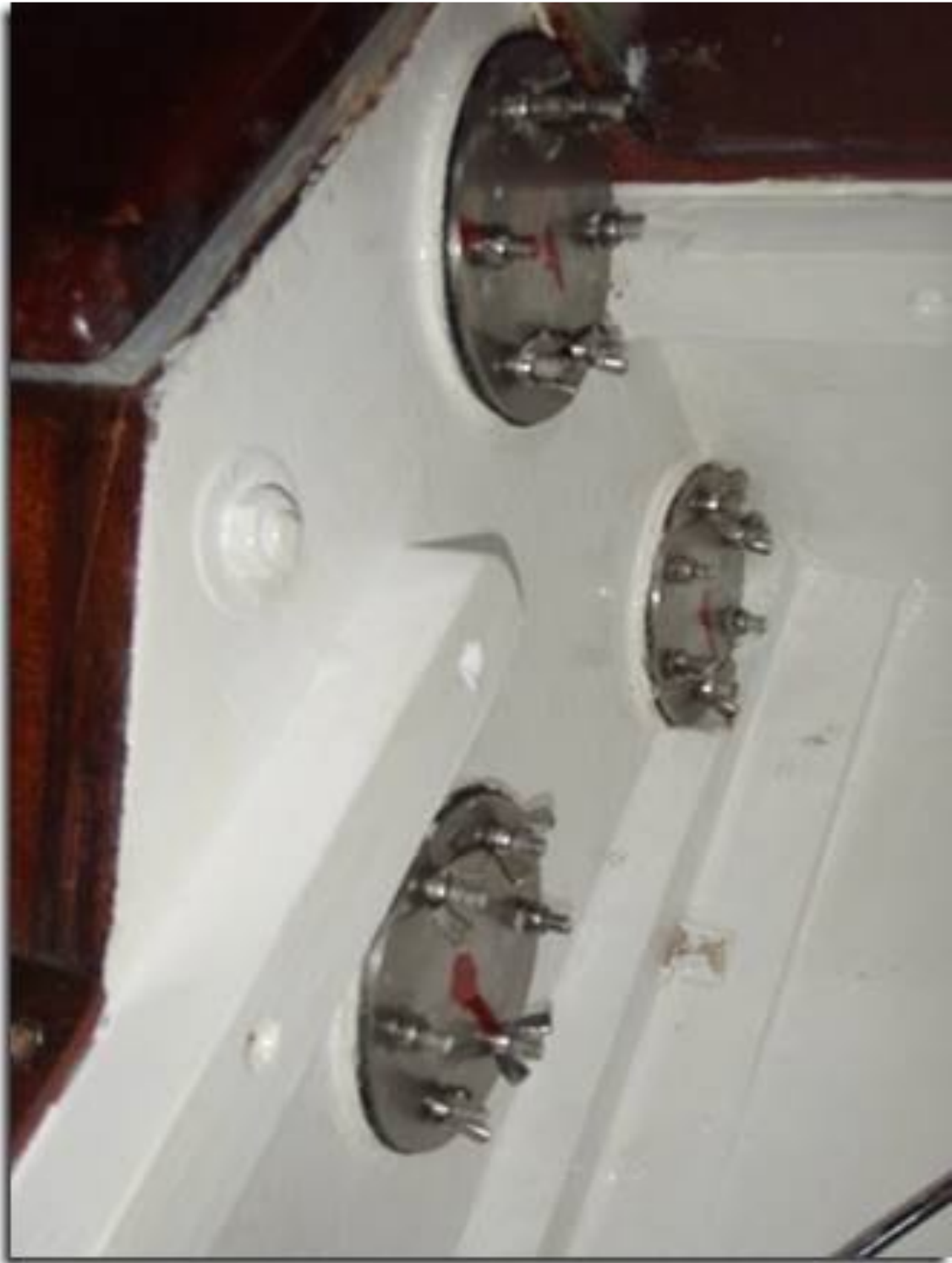
The completed installation. Slight misalignment of the welded set screws makes the covers individually paired to their bases. Hence the alignment marks.
